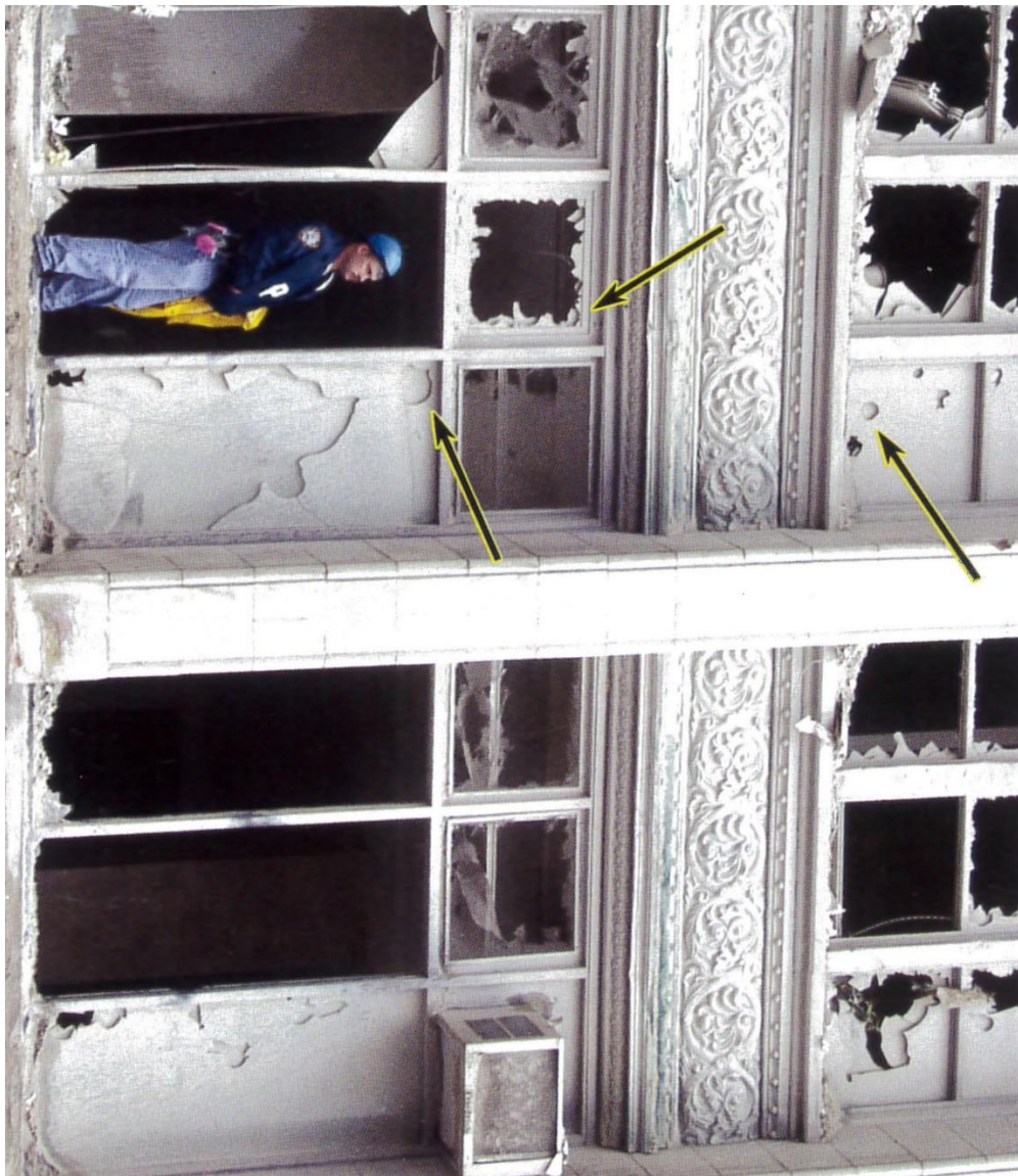
Figure 5 strange broken double planed windows
